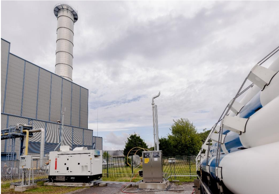
DEUTZ H2-Genset on the premises of RheinEnergie in Cologne Source: RheinEnergie AG
