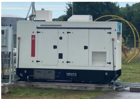
1. H2-GenSet in Pilotanwendung
