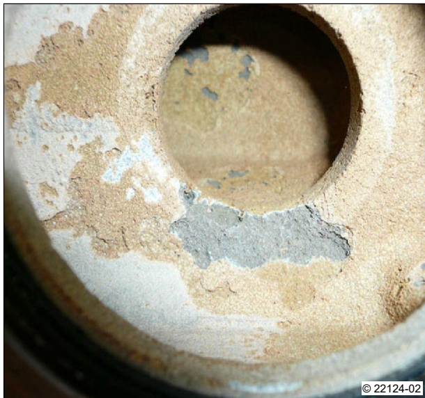
A12: Aluminium thermostat cover, corroded
