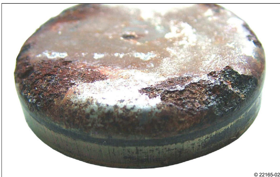
A11: Sealing cover, corroded
